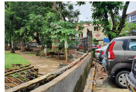
External fences in dilapidated condition
